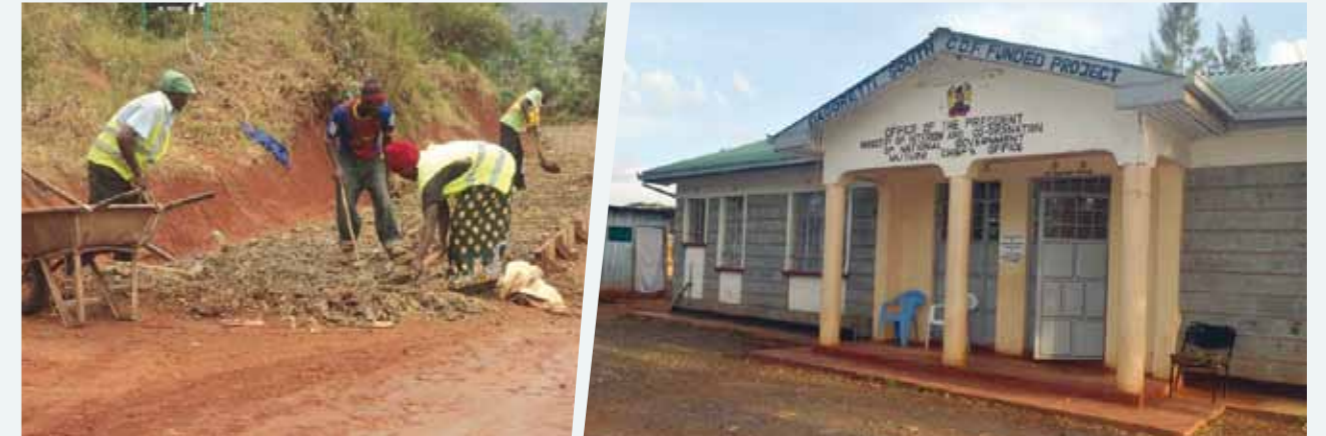
Road construction projects at Mukurweini constituency, Nyeri county. The programme is funded by the CDF kitty and the national government Dagoretti South Constituency - CDF Projects
